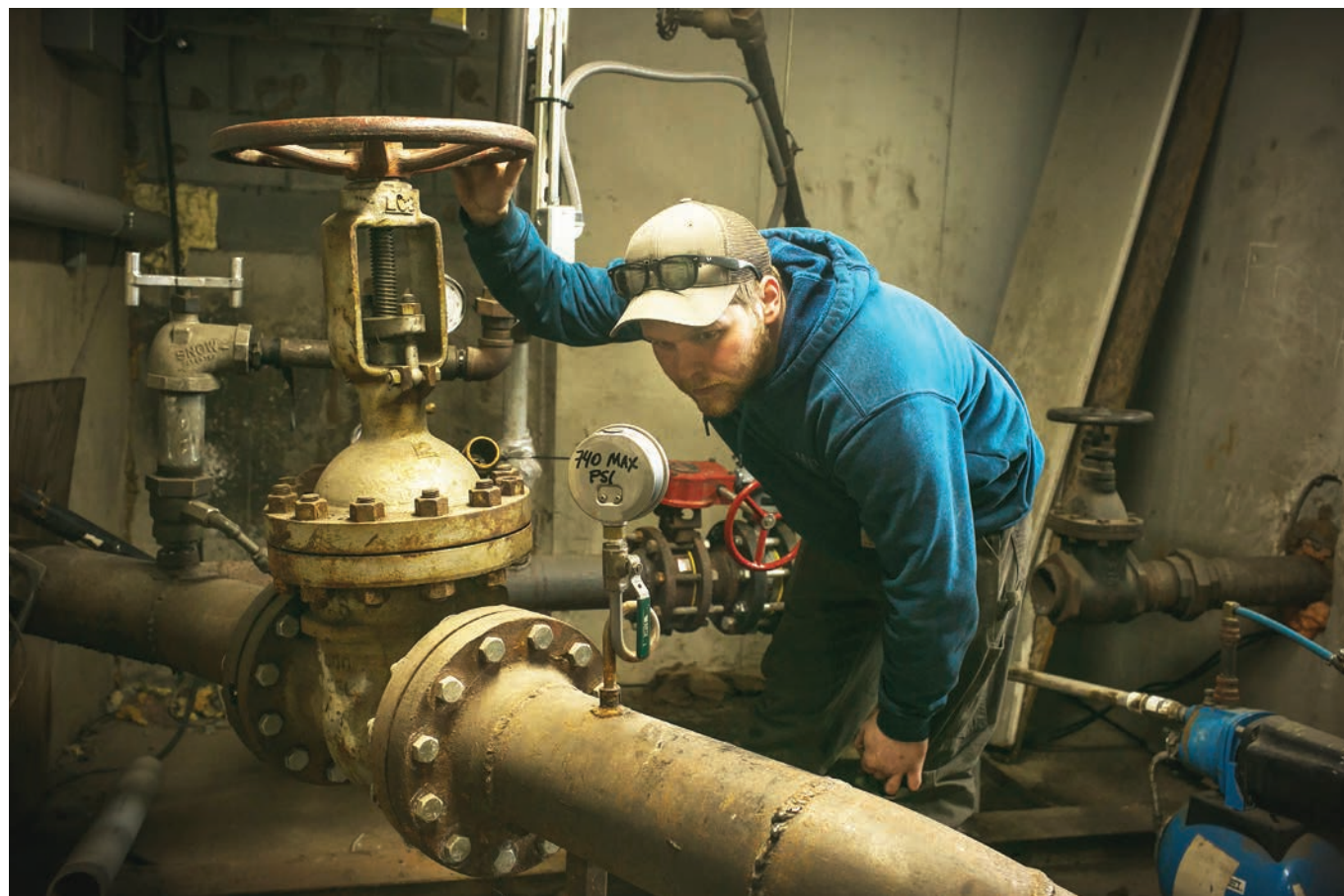
Snow-blowing manager Kevin Davie checks the water pressure in the pump house at the base of Plattekill Mountain. Plattekill has installed more than 28 miles of piping to pump water up the mountain for snowmaking.
